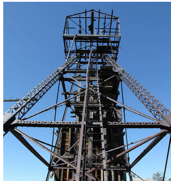
The "Eiffel" steel head frame at the Kelly Mine (New Mexico Historical photo)
